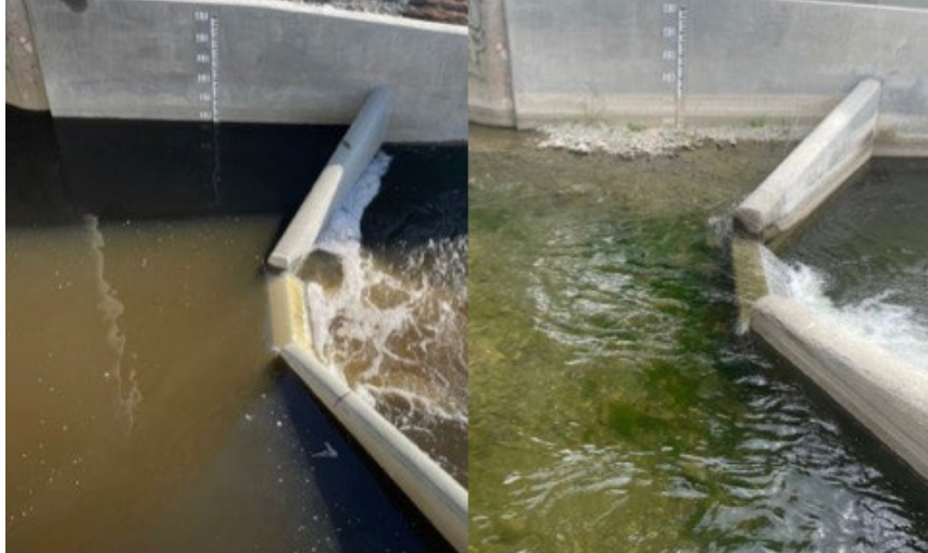
Figure 5-13. Demonstration of sediment deposited at the upstream extent of the RD1 lower ladder. Photo on the left was taken on 15 December 2022 and photo right was taken on 21 August 2023.
