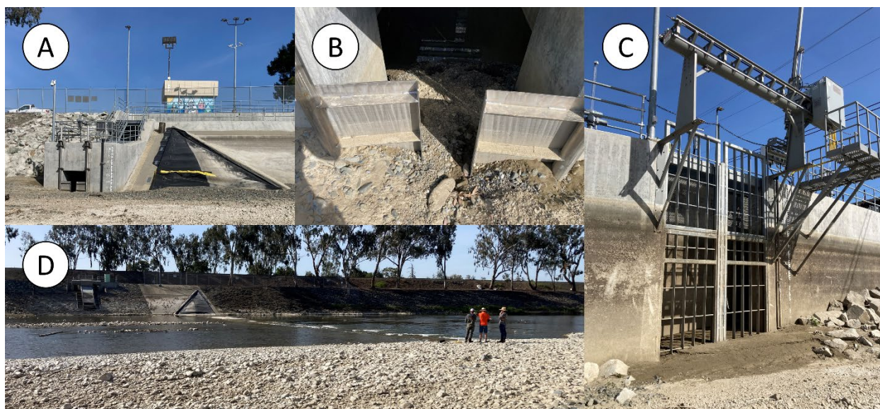
Figure 5-3: Sediment deposition at RD3 fish ladder. In clockwise order: A) entrance gate and river right side of buried RD3 dam apron; B) entrance gate buried in sediment; C) exit gate and trash rake; and D) dam apron with flow over top, buried in sediment.
