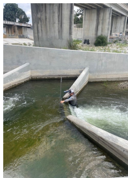
Figure 5-14: Site 4 in middle of lower fish ladder. Notice the large amounts of sediment on the downstream river left of the pool BHF is standing in. This sediment is blocking the weep holes which facilitate downstream juvenile migration.
